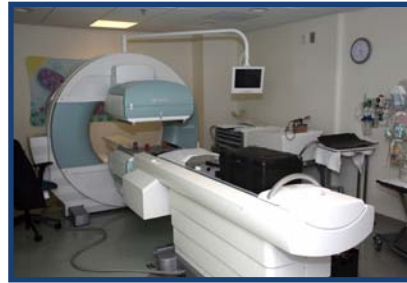
The assembly of a new Nuclear Medicine Suite will allow for more children to receive specialized care.
