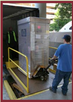
The PACS servers arrived in October and are in the first state of installation.
